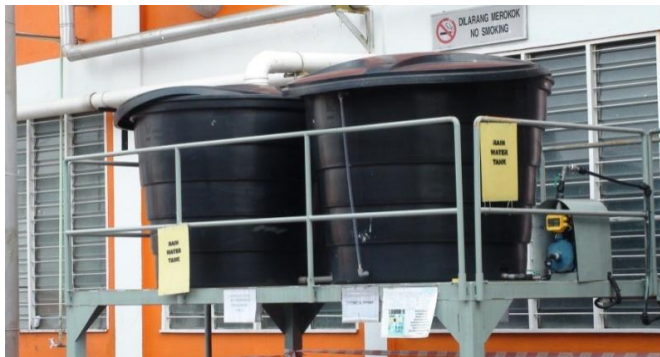
Rainwater harvesting by MM Vitaoils Sdn Bhd
