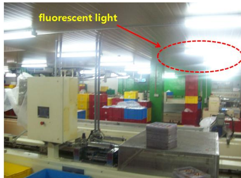
Use of inefficient lights
