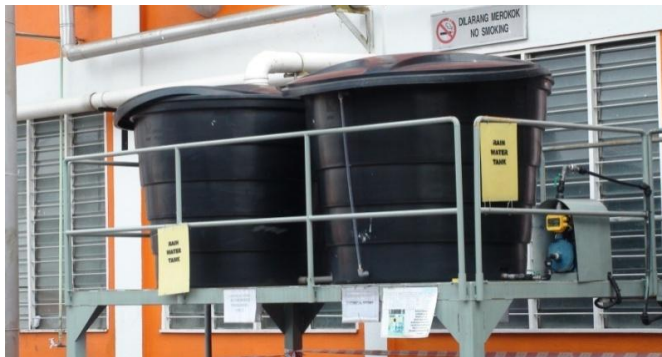
Rainwater harvesting by MM Vitaoils Sdn Bhd
