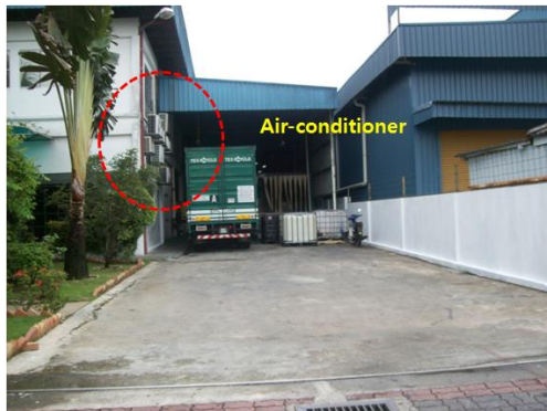
Independent air conditioning unit
