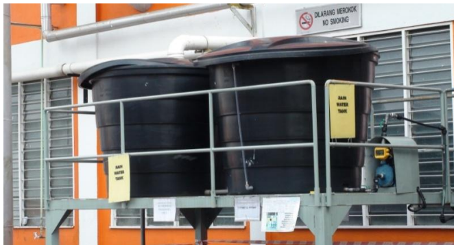
Rainwater harvesting by MM Vitaoils Sdn Bhd
