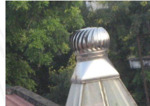
natural exhaust system.
