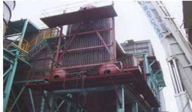
Generation steam by using tubular waste heat boiler
